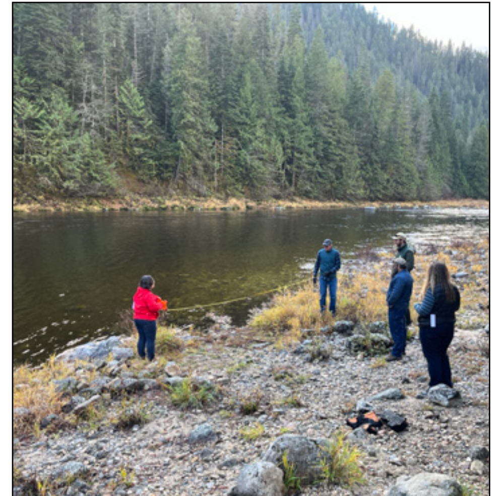
The USACE team takes measurements at Knife Edge, on the Lochsa, for the new boat ramp.
